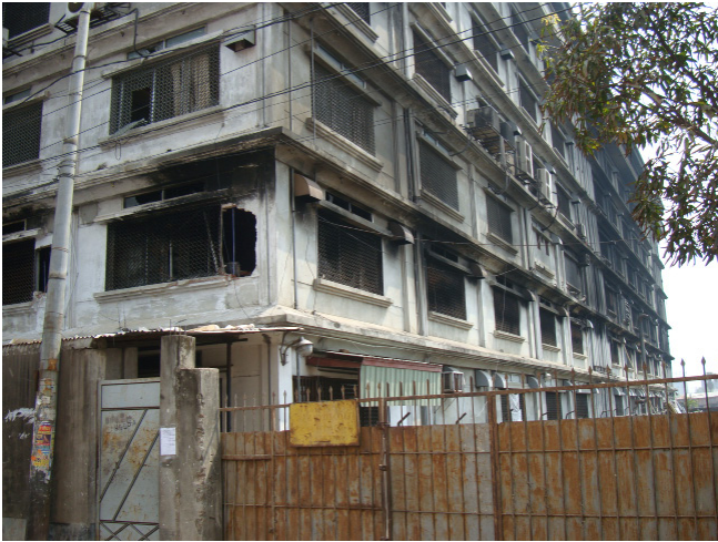
The fire started on the first floor of the Garib & Garib factory. Photo: BCWS.
